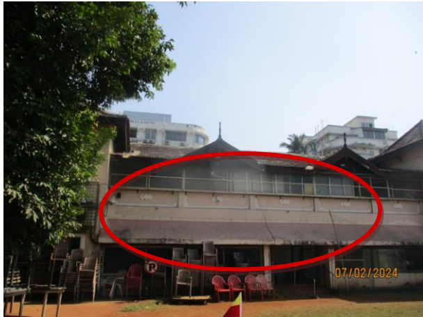
BLACK FUNGUS & CRACKS AT WALL PLASTER
