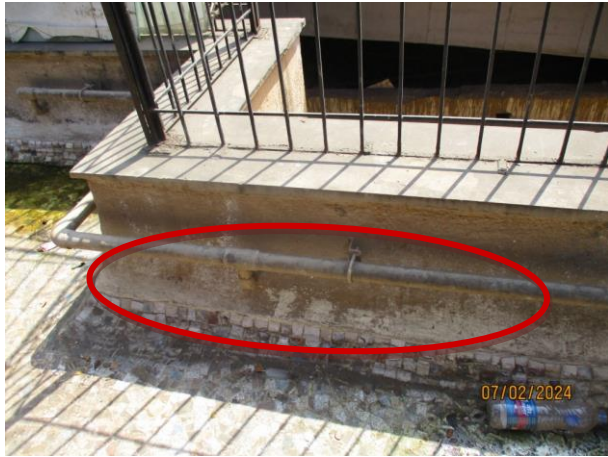
CRACKS AT CHINA CHIPS TOP SURFACE
