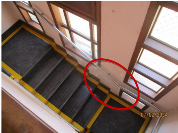
FLAKING OF PAINT AT WALL
