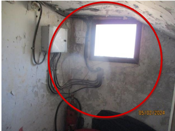
STAIRCASE BOTTOM AREA - CRACKS & FLAKING OF PAINT AT WALL
