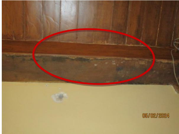
BANQUET HALL - SEEPAGE MARKS AT WOODEN CEILING
