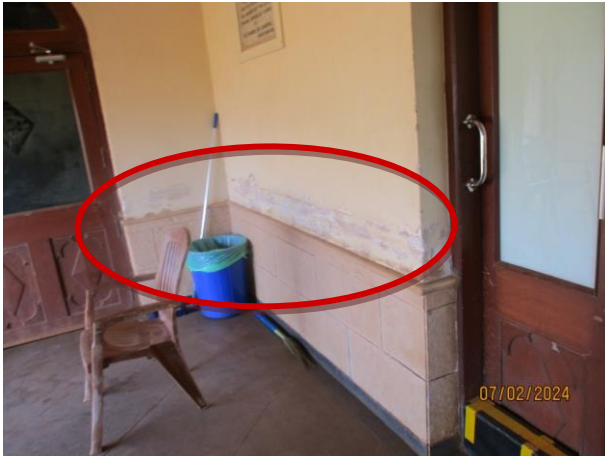
FLAKING OF PAINT AT WALL
