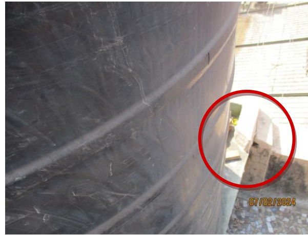
FINE CRACKS AT PLASTER
