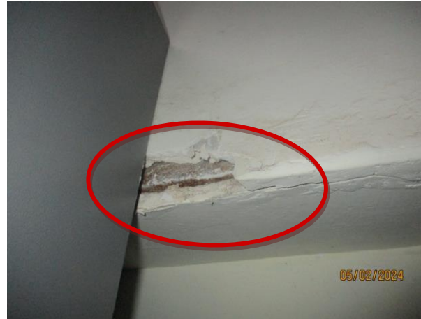
MEMBERS LOCKER ROOM - CRACKS AT BEAM CORRODED STEEL BARS EXPOSED
