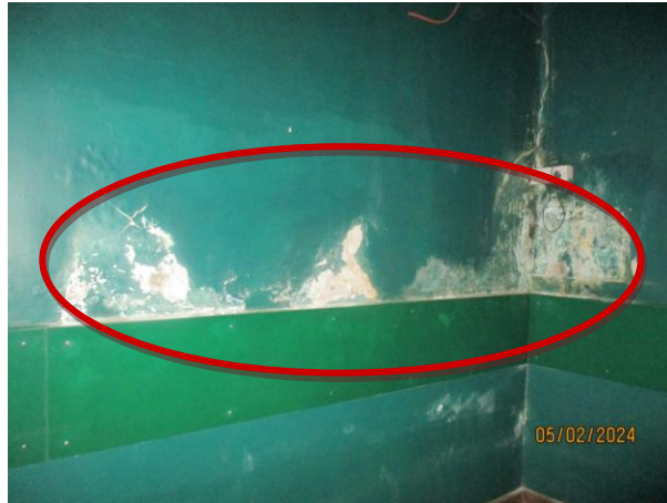
BADMINTON ROOM - FLAKING OF PAINT AT WALL
