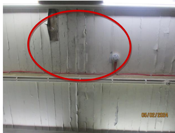
BADMINTON ROOM - CRACKS & LOOSE PAINT AT WOODEN ROOF AREA S
