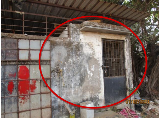
CRACKS AT EXTERNAL WALL PLASTER
