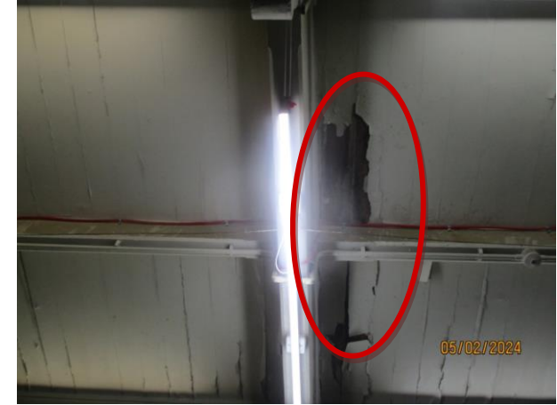
BADMINTON ROOM - BAD CONDITION OF ROOF AREA
