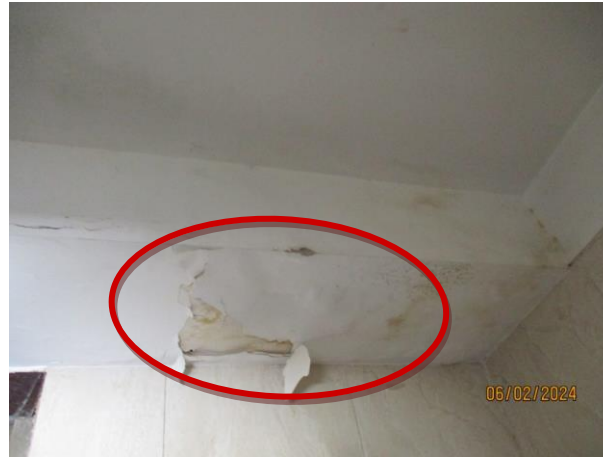
TOILET - FLAKING OF PSINT AT CEILING
