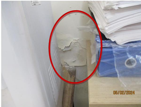
GYMKHANA OFFICE - FLAKING OF PAINT AT WALL
