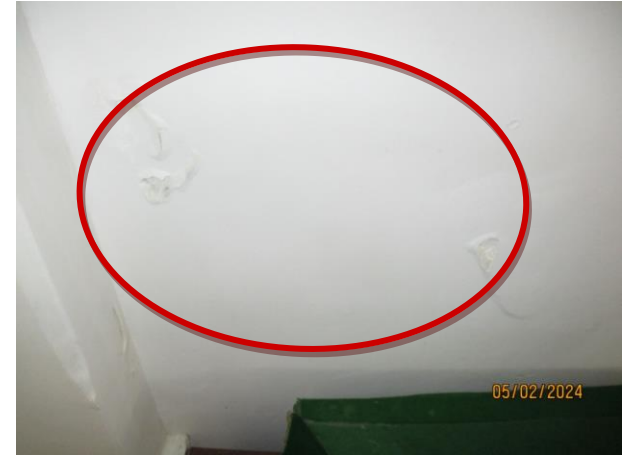
BILLIARD ROOM - PAINT PEELING AT CEILING
