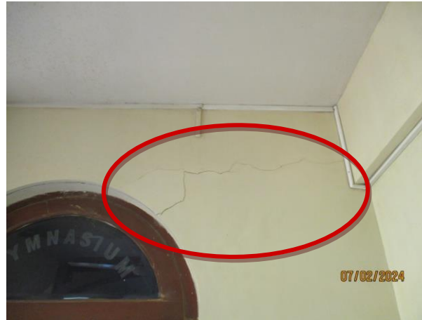
CRACKS AT WALL
