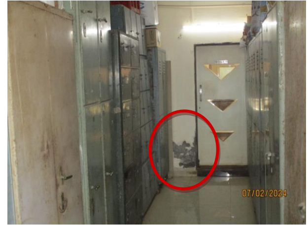
CRACSK & FLAKING OF PAINT AT WALL
