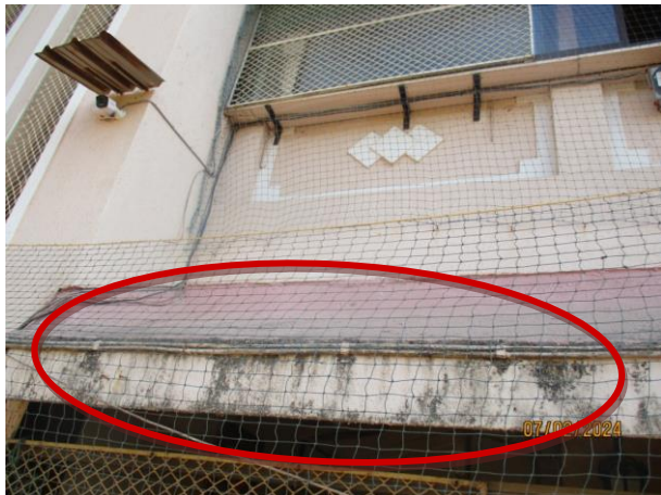
BLACK FUNGUS AT WALL PLASTER
