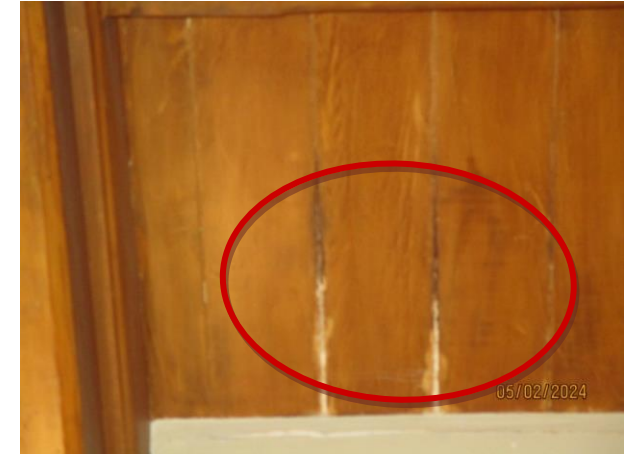
BANQUET HALL - SEEPAGE MARKS AT WOODEN CEILING
