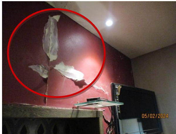
SILLY POINT (BAR) - FLAKING OF PAINT AT WALL
