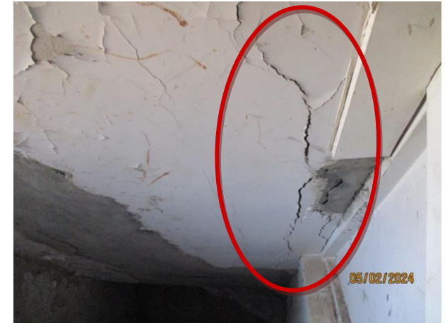
STAIRCASE BOTTOM AREA - CRACKS AT CEILING
