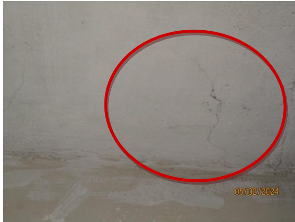
GYMKHANA OFFICE - CRACKS AT CEILING
