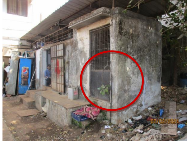
VEGETATION GROWTH FROM WALL
