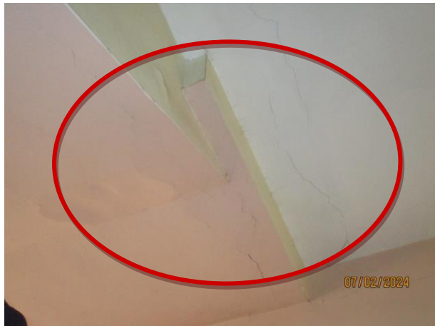
CRACKS AT CEILING
