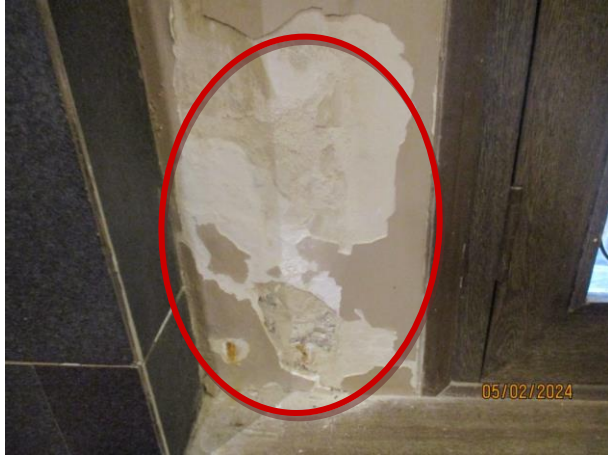
CLEAN BOWL (DINING ROOM) - FLAKING OF PAINT AT WALL
