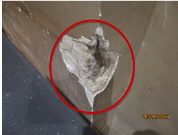
SILLY POINT (BAR) - DISTRESS AT COLUMN
