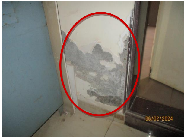
TOILET - FLAKING OF PAINT AT WALL
