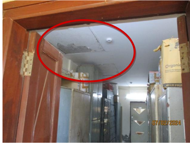
FLSKING OF PAINT AT CEILING
