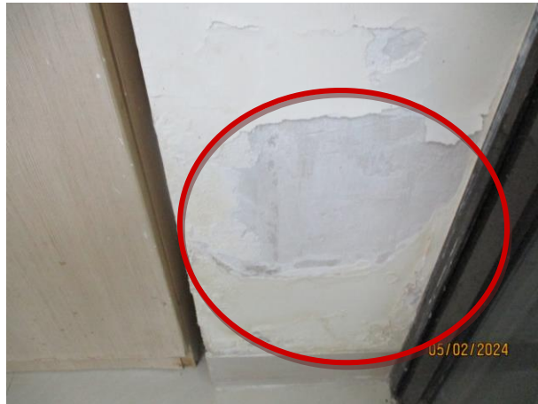
GYMKHANA OFFICE - FLAKING OF PAINT AT WALL
