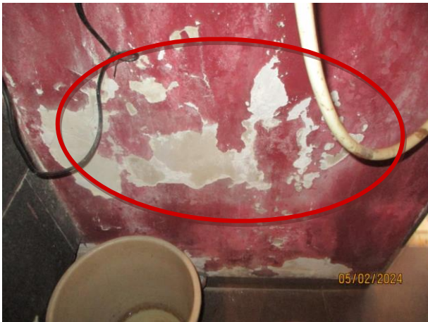
SILLY POINT (BAR) - FLAKING OF PAINT AT WALL
