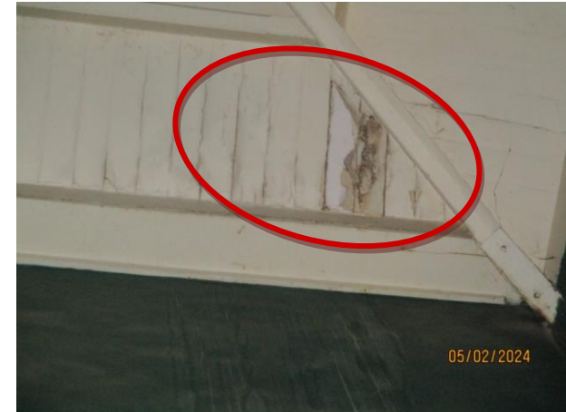
BADMINTON ROOM - WOODEN ROOF FOUND IN ROTTEN CONDITION
