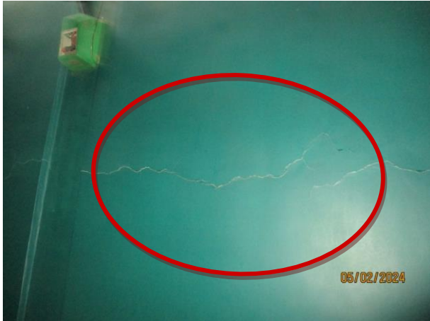
BADMINTON ROOM - CRACKS AT WALL PLASTER
