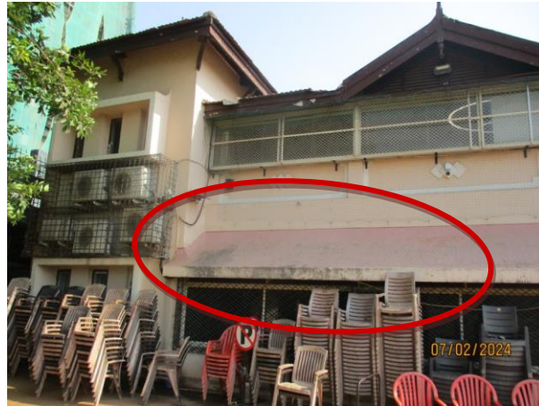
BLACK FUNGUS & CRACKS AT WALL PLASTER
