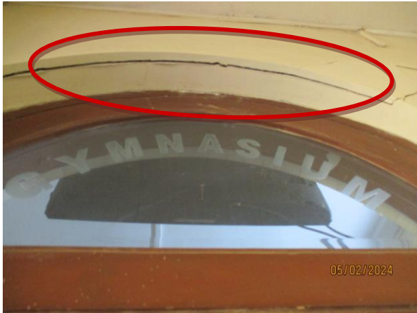
GYMNASIUM - CRACKS AT WALL
