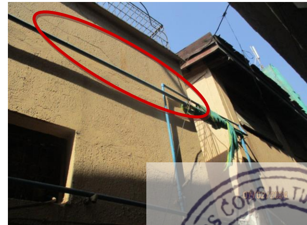
CRACKS AT WALL PLASTER
