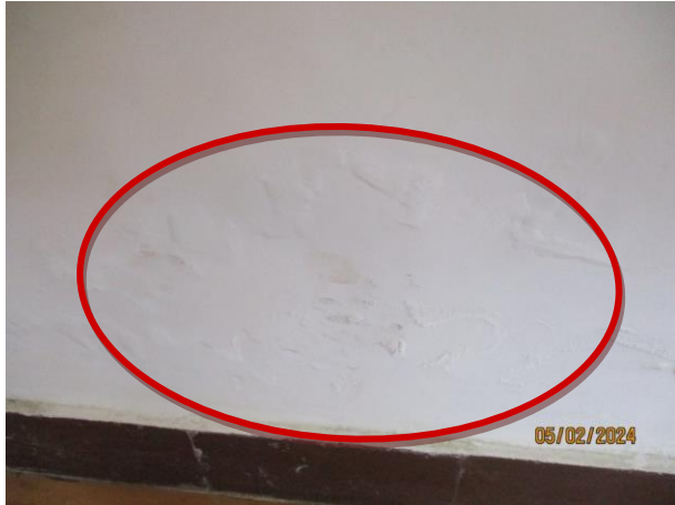
BILLIARD ROOM - FLAKING OF PAINT AT WALL
