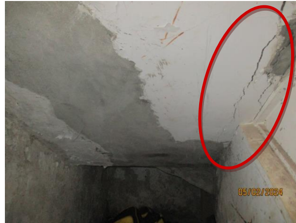
STAIRCASE BOTTOM AREA - CRACKS AT CEILING
