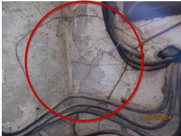
STAIRCASE BOTTOM AREA - FLAKING OF PAINT AT WALL
