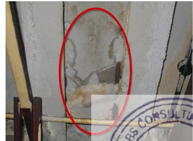
CLEAN BOWL (DINING ROOM) - SEEPAGE MARKS & PAINT PEELING AT CEILING
