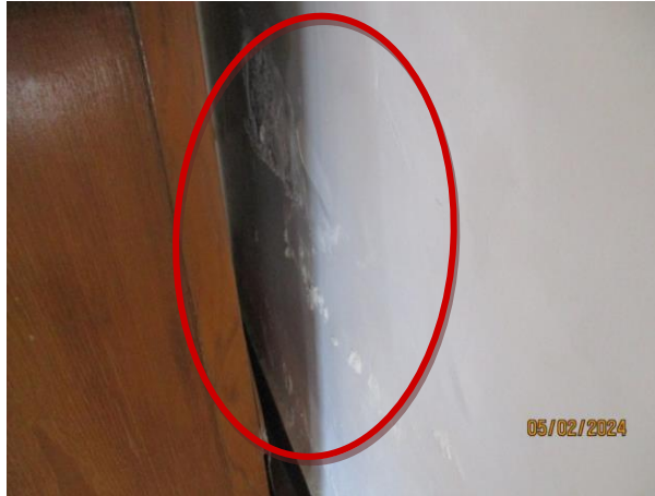
BILLIARD ROOM - FLAKING OF PAINT AT WALL
