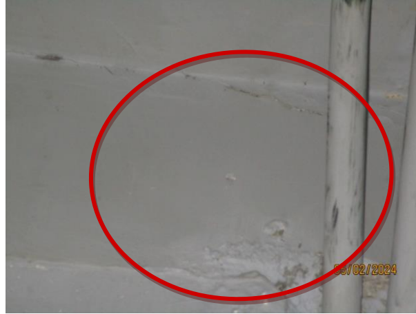
CLEAN BOWL (DINING ROOM) - CRACKS & FLAKING OF PAINT AT WALL & CEILING
