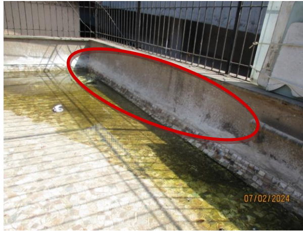
CRACKS AT PARAPET WALL PLASTER
