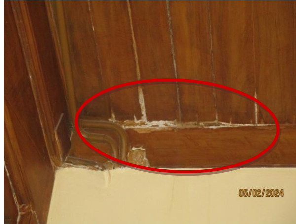
BANQUET HALL - SEEPAGE MARKS AT WOODEN CEILING
