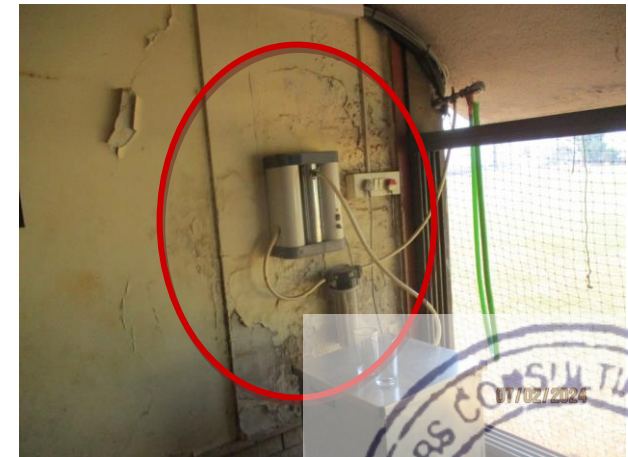
FLAKING OF PAINT AT WALL
