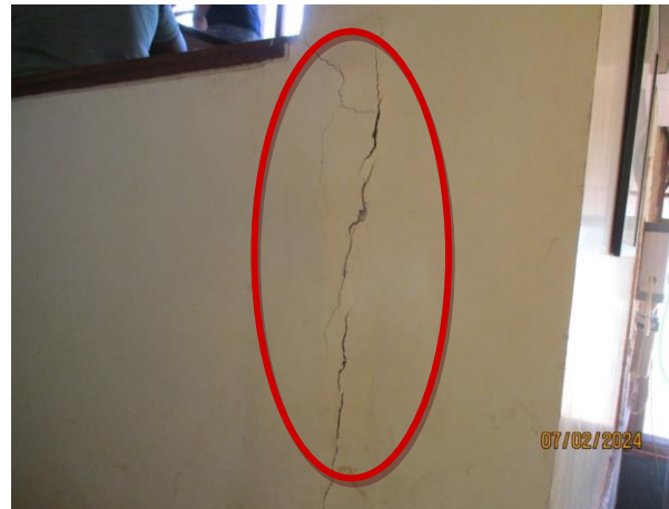
CRACKS AT WALL
