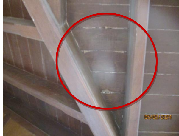
CARD ROOM - JOINTS ARE OPEN BETWEEN WOODEN PLANKS
