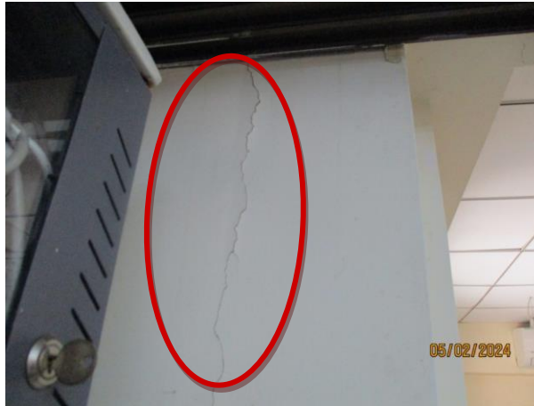
GYMKHANA OFFICE - CRACKS AT WALL
