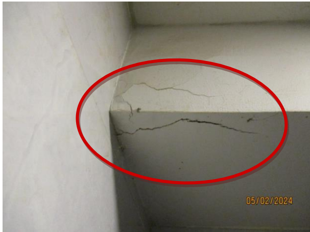
MEMBERS LOCKER ROOM - CRACKS AT BEAM BOTTOM
