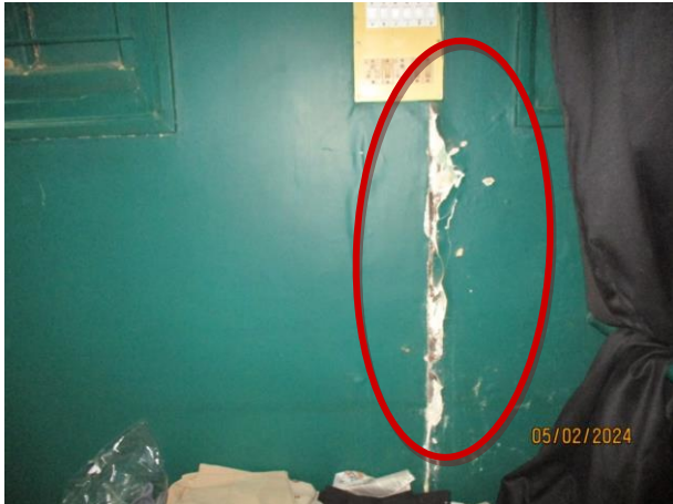
BADMINTON ROOM - FLAKING OF PAINT AT WALL
