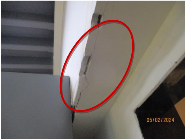
MEMBERS LOCKER ROOM - CRACKS AT BEAM
