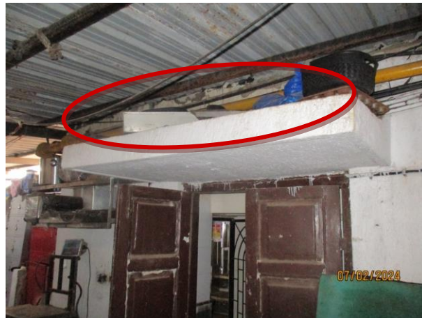
CRACKS AT WALL PLASTER
