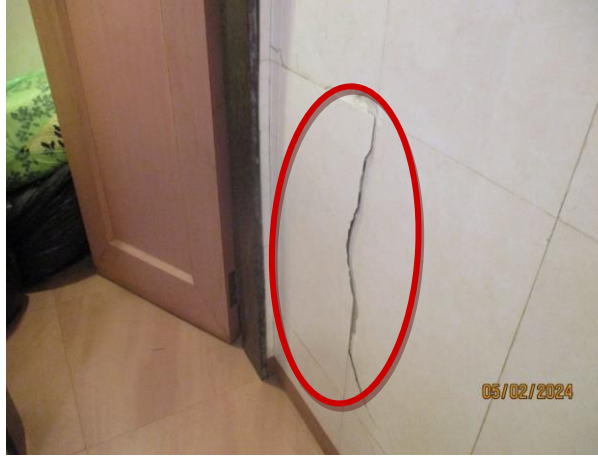
BADMINTON ROOM - CRACKS AT WALL PAINT
