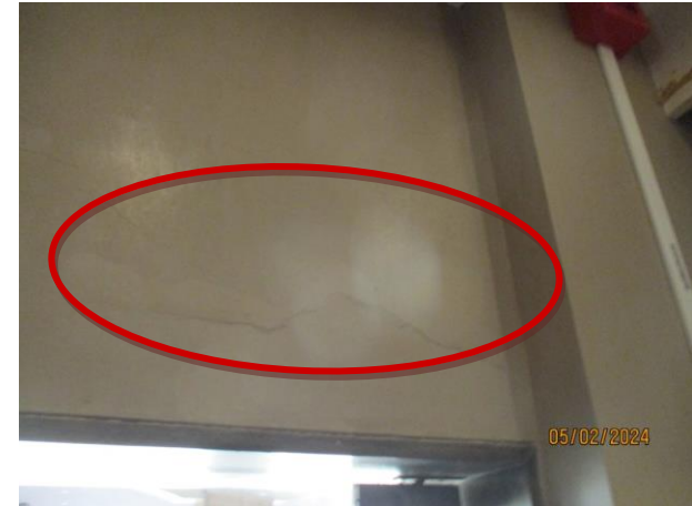
SILLY POINT (BAR) - CRACKS AT WALL
