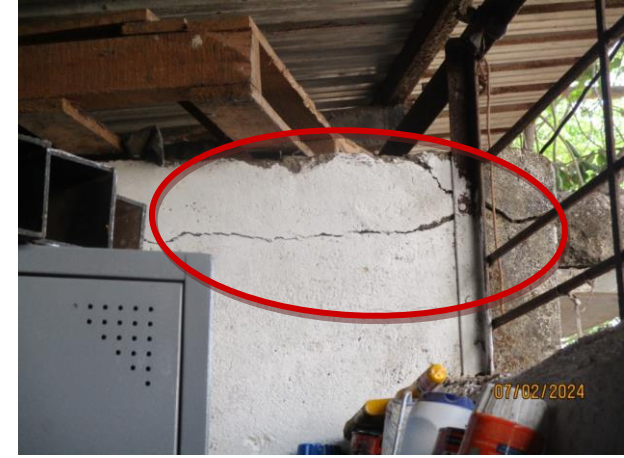
CRACKS AT WALL
