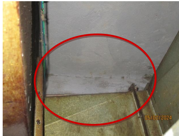
CLEAN BOWL (DINING ROOM) - FLAKING OF PAINT AT CEILING
