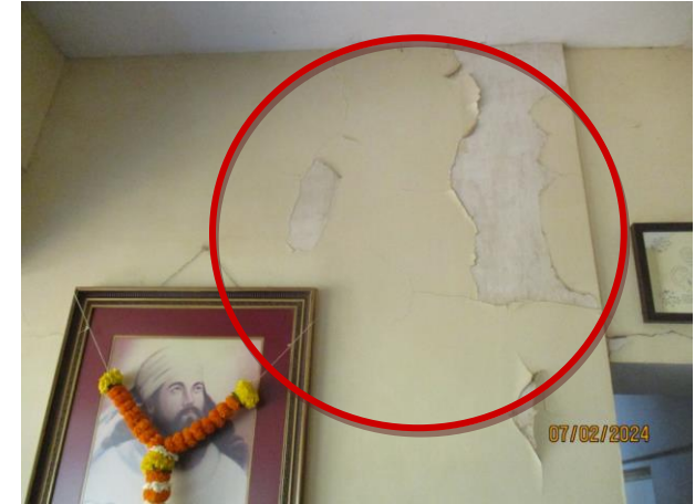
FLAKING OF PAINT AT WALL
