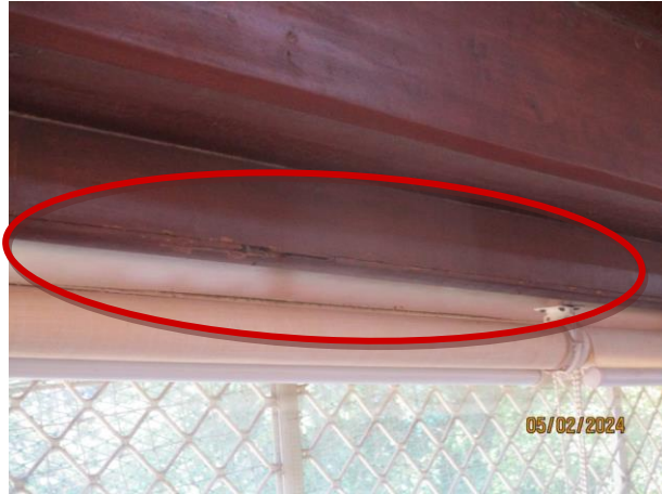
CARD ROOM - CRACKS AT LINTEL BEAM PLASTER
