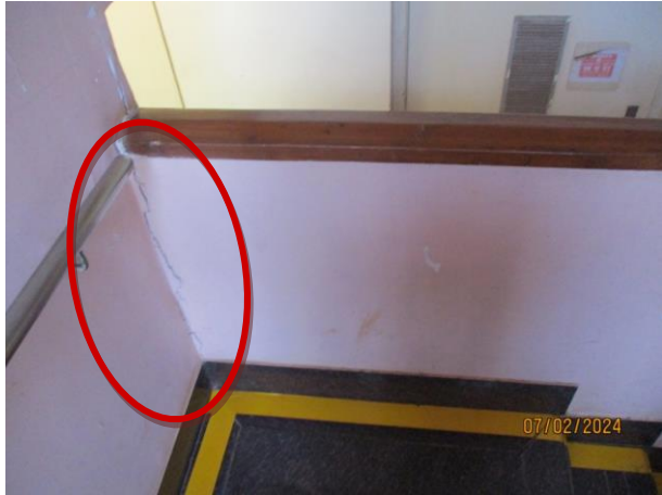
CRACKS AT WALL PLASTER
