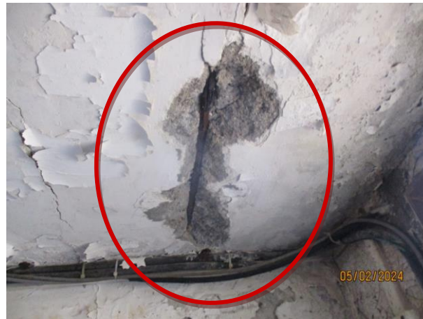
STAIRCASE BOTTOM AREA - CORRODED STEEL BARS EXPOSED AT CEILING
