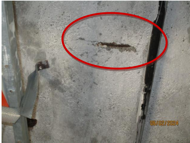
TOILET - CORRODED STEEL BARS EXPOSED AT CEILING
