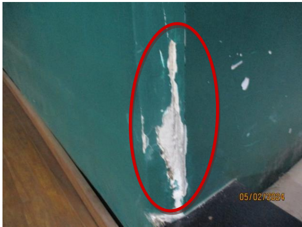
BADMINTON ROOM - FLAKING OF PAINT AT WALL
