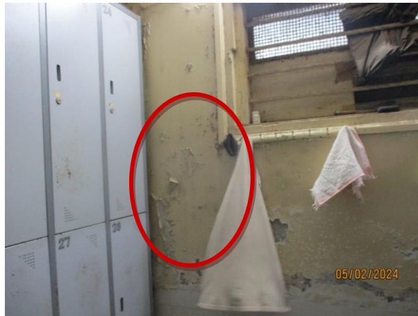
BADMINTON ROOM - FLAKING OF PAINT AT WALL
