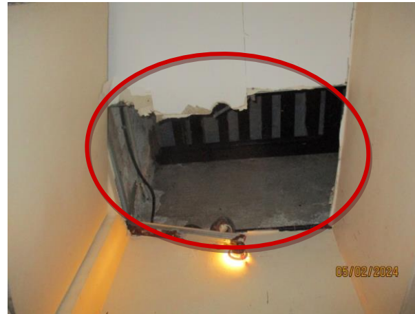
MEMBERS LOCKER ROOM - DAMAGED FALSE CEILING OBSERVED
