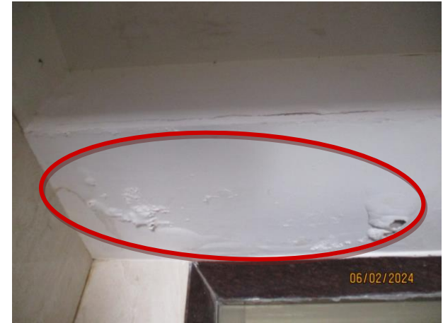
TOILET - FLAKING OF PAINT AT CEILING
