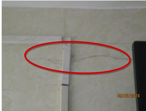
GYMNASIUM - CRACKS AT WALL
