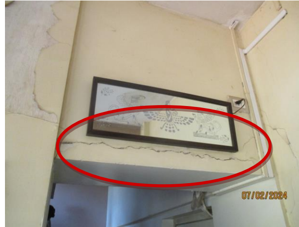
CRACKS AT BEAM
