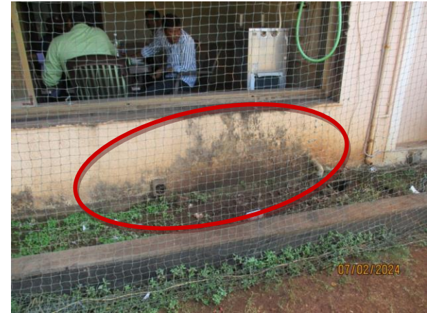
BLACK FUNGUS AT WALL PLASTER
