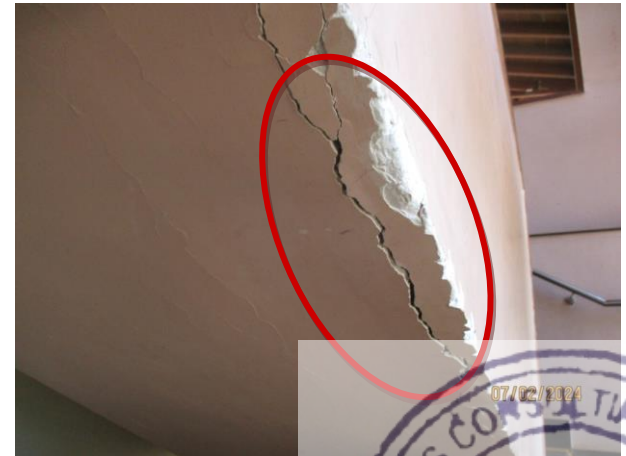
CRACKS AT CEILING PLASTER
