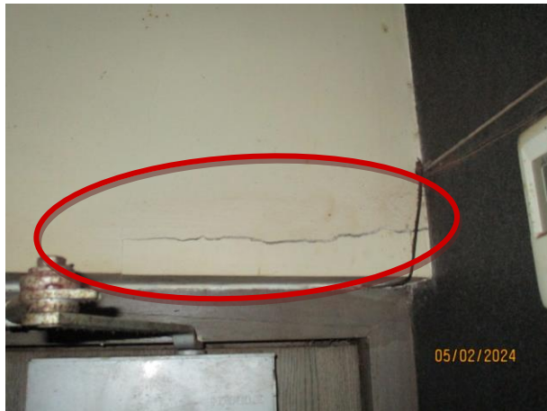
CLEAN BOWL (DINING ROOM) - CRACKS AT WALL
