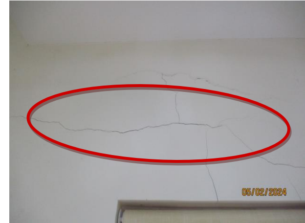
CARD ROOM - MULTIPLE CRACKS AT WALL PLASTER
