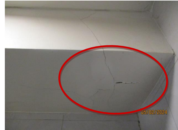
MEMBERS LOCKER ROOM - CRACKS AT BEAM BOTTOM
