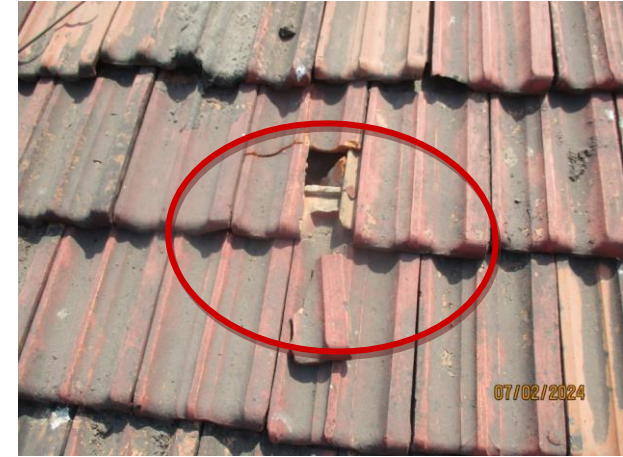
MANGLORE TILES FOUND DAMAGED
