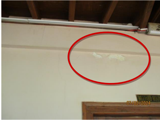
FLAKING OF PAINT AT WALL
