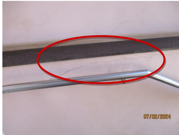
CRACKS AT WALL
