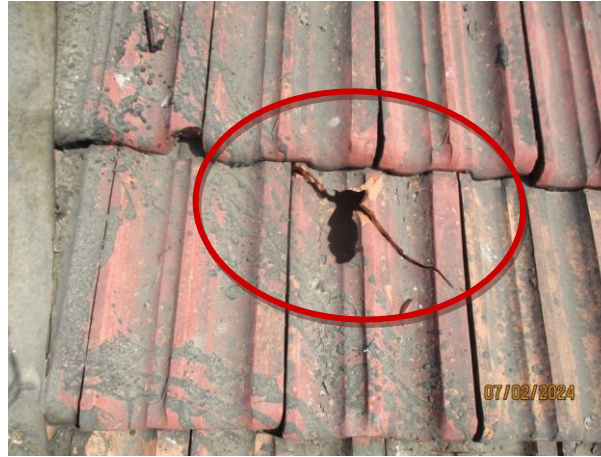
MANGLORE TILES FOUND DAMAGED
