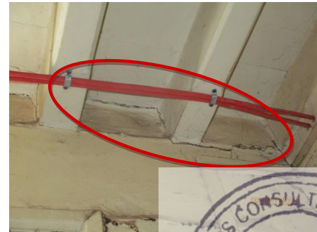
BADMINTON ROOM - CRACKS AT WALL PLASTER
