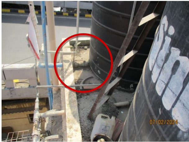
VEGETATION GROWTH FROM AT PLUMBING LINES
