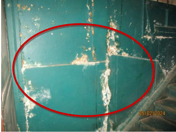
BADMINTON ROOM - FLAKING OF PAINT AT WALL
