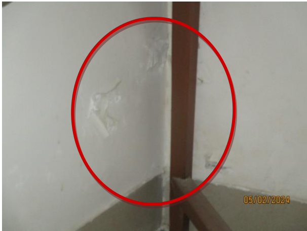
CARD ROOM - FLAKING OF PAINT AT WALL
