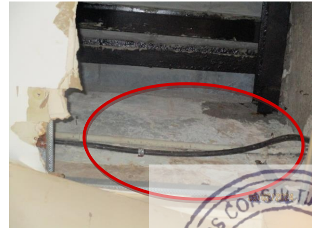
MEMBERS LOCKER ROOM - FLAKING OF PAINT AT WALL
