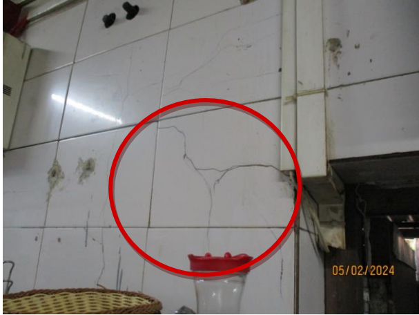
CLEAN BOWL (DINING ROOM) - CRACKS AT WALL TILES
