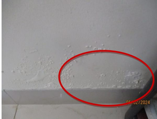
SECRETARY OFFICE - PAINT PEELING AT WALL
