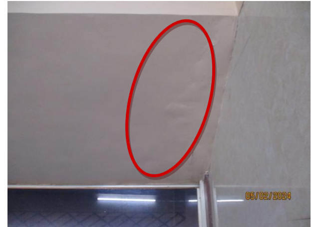
GYMNASIUM - FLAKING OF PAINT AT CEILING
