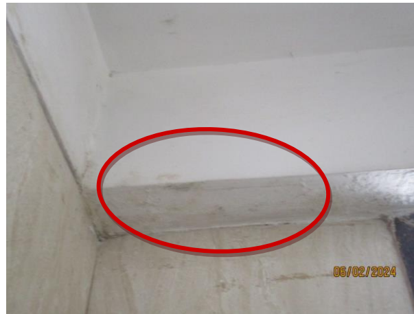
TOILET - FLAKING OF PAINT AT WALL
