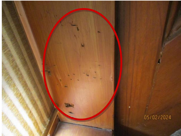
BANQUET HALL - BAD CONDIRION OF CEILING
