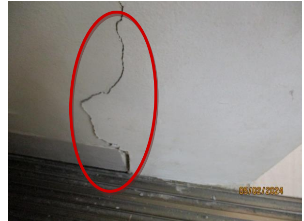
GYMKHANA OFFICE - CRACKS AT WALL
